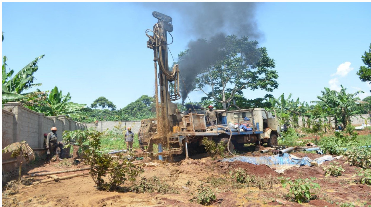
Figure 7: In order to solve the high water bills at Home of Hope, it was necessary to drill a water point for safe and cheap water supply.
